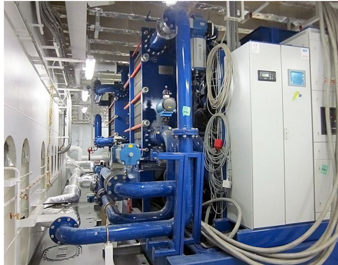
Figure 18 Opcon Powerbox ORC Marine version installed inside the engine room of “MV Figaro”
