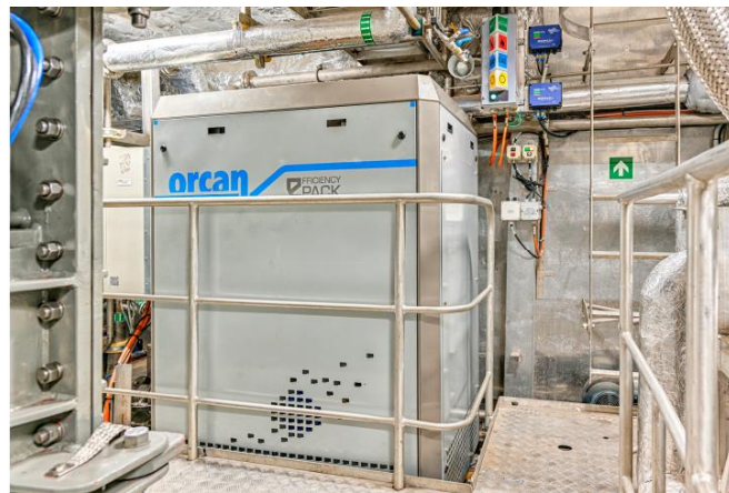
Figure 17 Orcan-Energy 'Efficiency Pack' installed inside the engine room of "MS Willem Barentsz"
