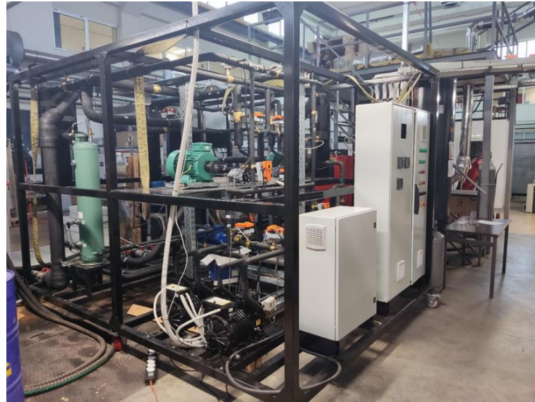
Figure 18 – Photograph of the ORC–ejector integrated heat pump prototype installed at the National Technical University of Athens .
