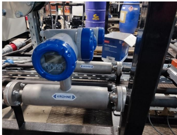
Figure 25 – Photograph of the Coriolis flow meters installed on the ORC–ejector integrated heat pump prototype.
