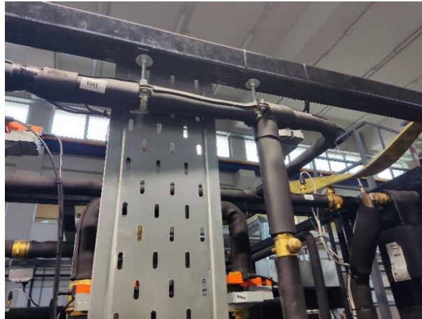
Figure 24 – Photograph of the thermally insulated ejector installed on the ORC–ejector integrated heat pump prototype.
