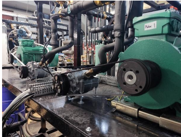
Figure 20 – Photograph of the expanders and motors installed on the ORC–ejector integrated heat pump prototype.
